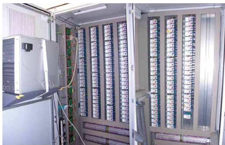
Fig. 6: The inside of the switch cabinet in the measuring technology and control room with more than 160 DC measurement amplifiers and the computer containing A/D converters
